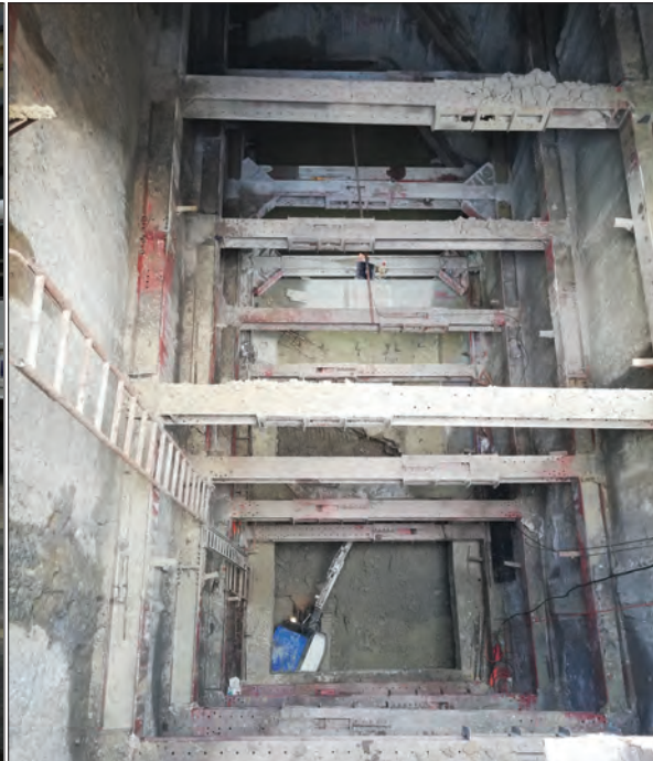
View of the Shaft 1 site with and without its steel decking cover
