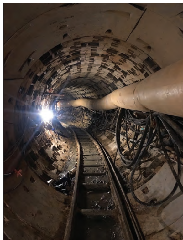
Transition between traditional lining rings and the short steel sets used in the Tunnel C tight radius curve
